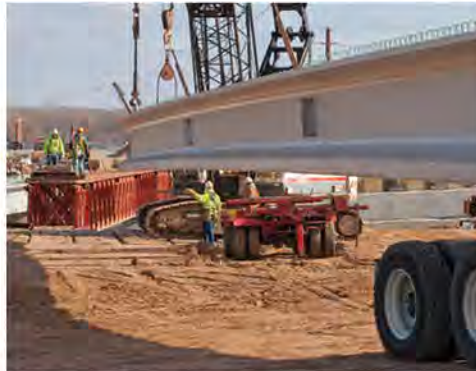
The final girders of the I-41 Project were set in place on the bridge over Duck Creek in April 2016.
