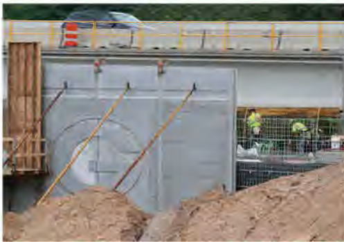
An example of Community Sensitive Solutions being installed at the Lombardi Avenue interchange.
